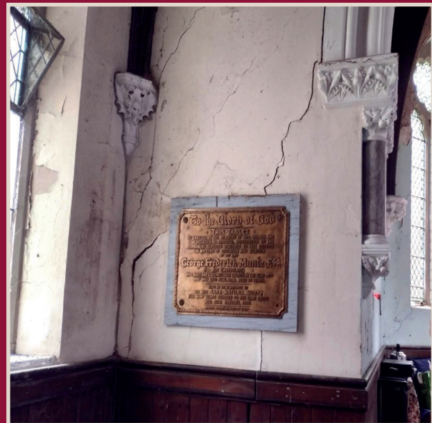
There are significant cracks requiring repair at Umberslade. Photo courtesy Kathryn Moore
